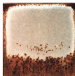
Galvanised steel Z275 (Heavy sign of Rust)
